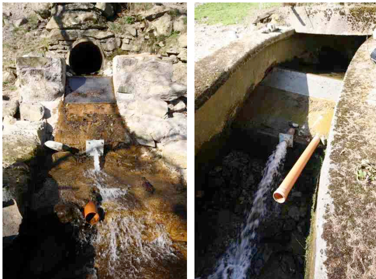
The two intakes, which supply the forebay tank
