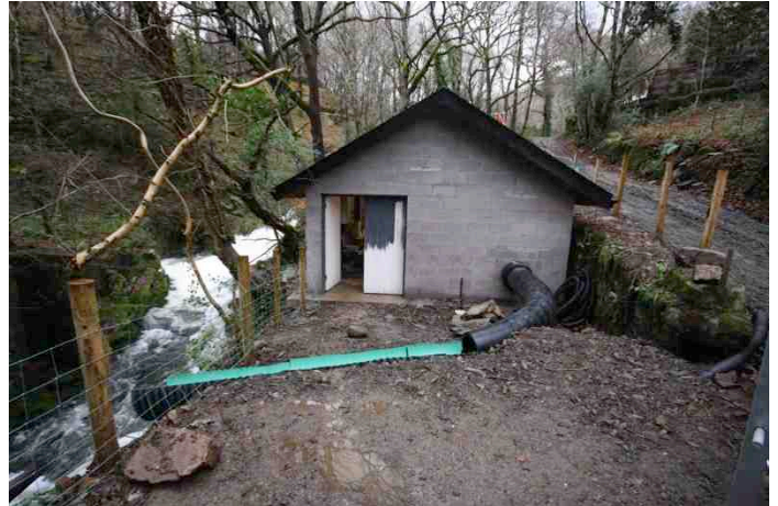
The powerhouse during construction showing the 'pigging' route. It is due to be clad in stone.
