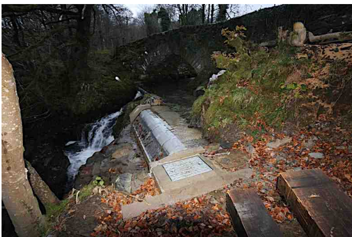
The intake weir which uses a coanda screen
